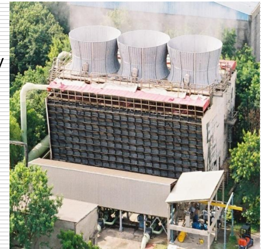
Conventional Type Cooling Tower
