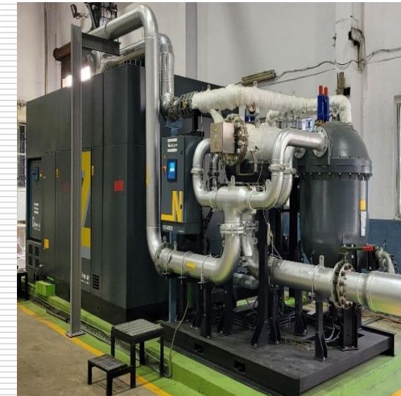
Centralized single Centrifugal Compressor
