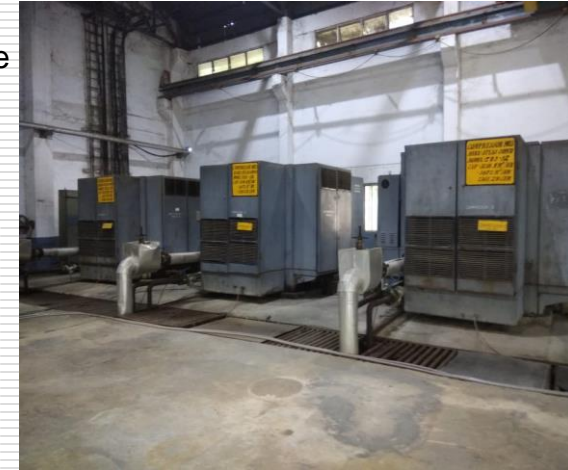
Old Screw Compressors – 3 Nos
